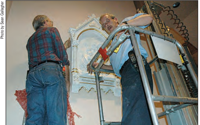
On April 5, from left, Don Huffman and Dan Wyrick, archdiocesan maintenance technicians, hang a depiction of Veronica wiping the face of Jesus in SS. Peter and Paul Cathedral in Indianapolis. It is a part of the Stations of the Cross that had previously hung in Assumption Church in Indianapolis. That parish closed on Dec. 31, 1994.
