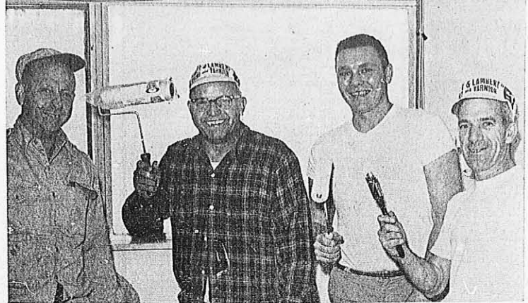
HELP REFURBISH RETREAT HOUSE WING—These four men were part of an army of 108 retreat captains and friends who pitched in on a recent Saturday morning and painted the interior walls of the "new" wing at Alverna Retreat House, Indianapolis. The entire job, carried out under the direction of Father Donald Paulus, Retreat House director, took only three hours and a half. Brandishing the weapons above are, left to right: Melf Doyle, Lou McFadden, Dick Warfield and Ray Laker.
